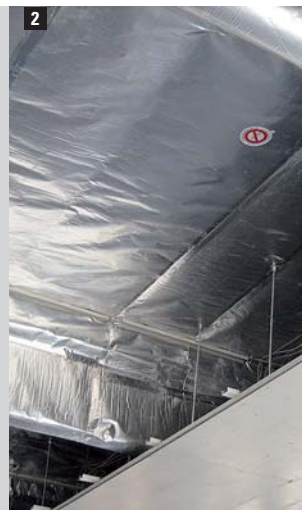
1/2 Fitting a vapour barrier and a Sisalex™ 514 air seal in a swimming pool.
